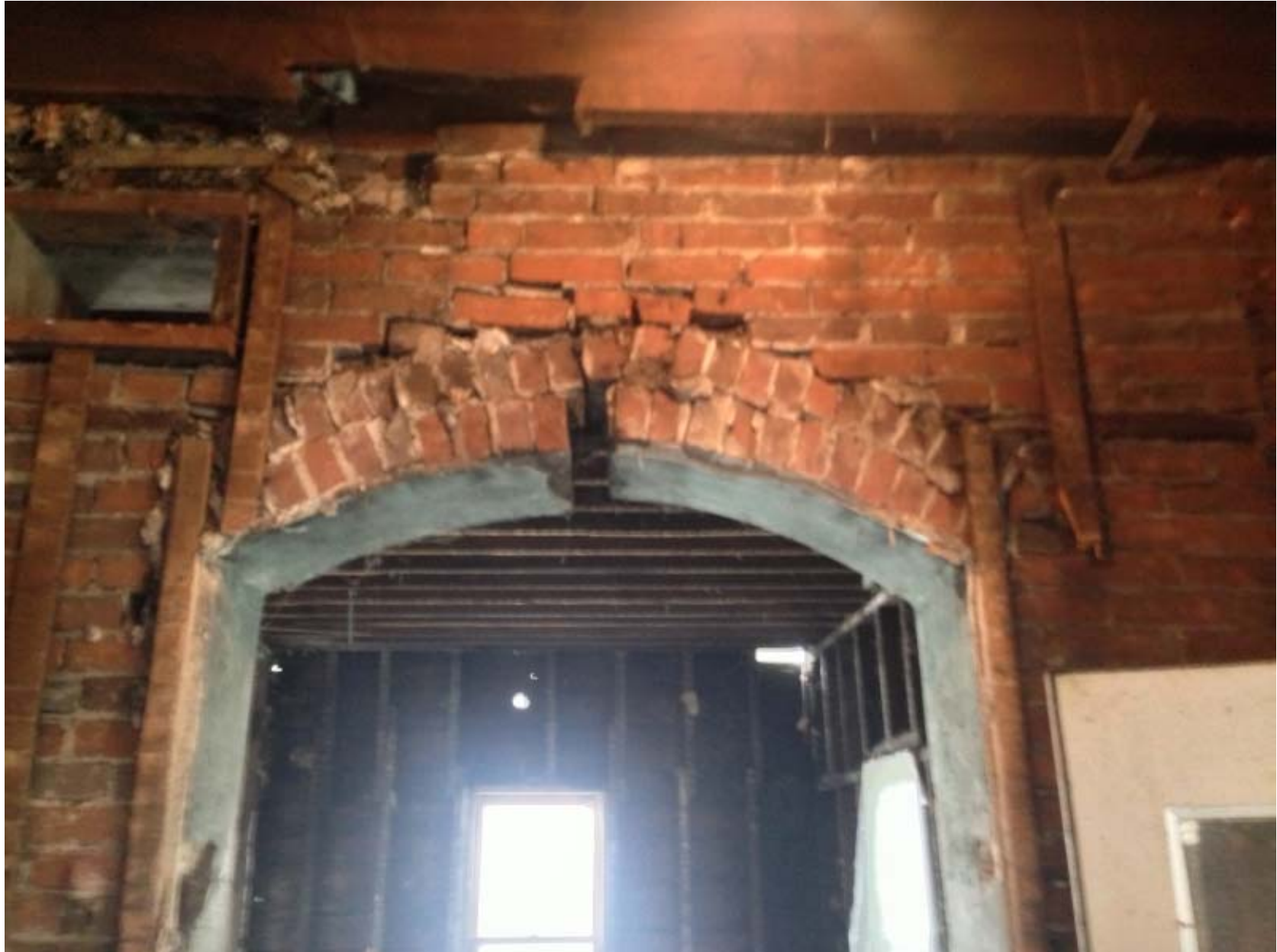
400 E. 22 nd Street – Example of Interior Cracks
