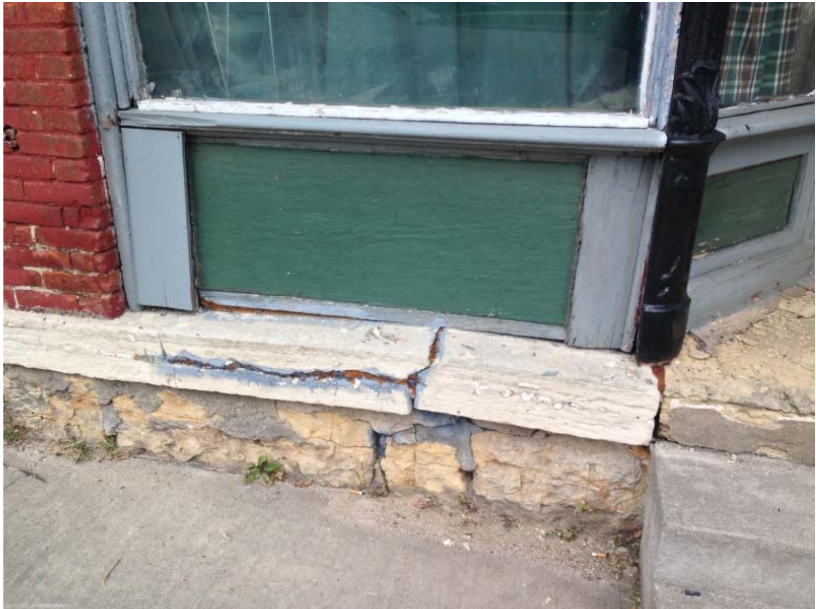
400 E. 22 nd Street – Example of Foundation Cracks
