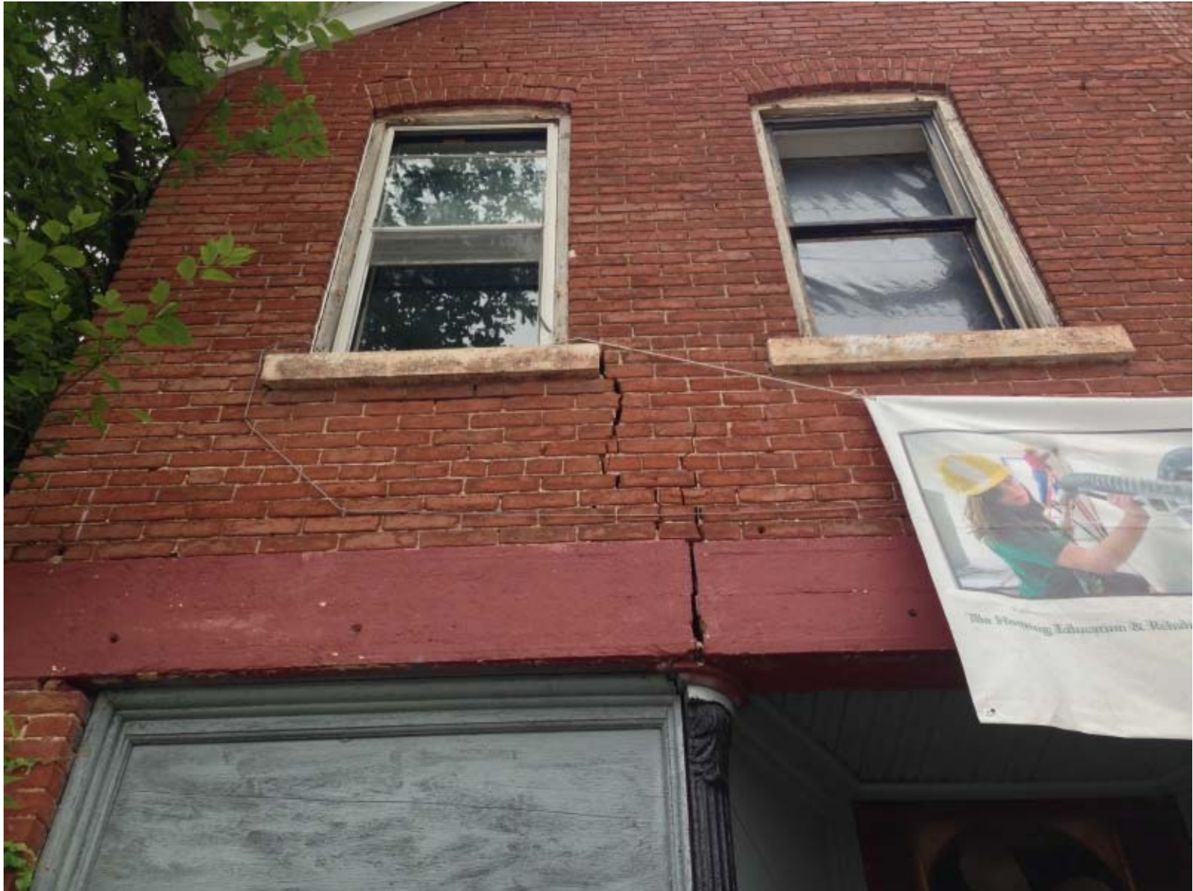
400 E. 22 nd Street – Example of Exterior Cracks
