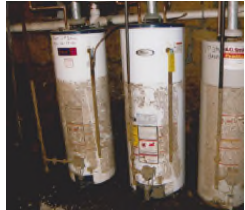
Basement flooding high water mark on water heaters
