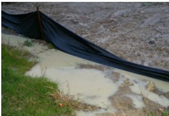
Silt fence failure allowing sediment to leave a construction site
