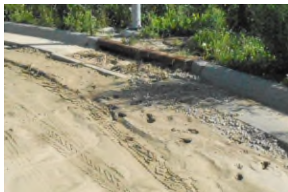
Sediment deposition clogging a storm sewer inlet
