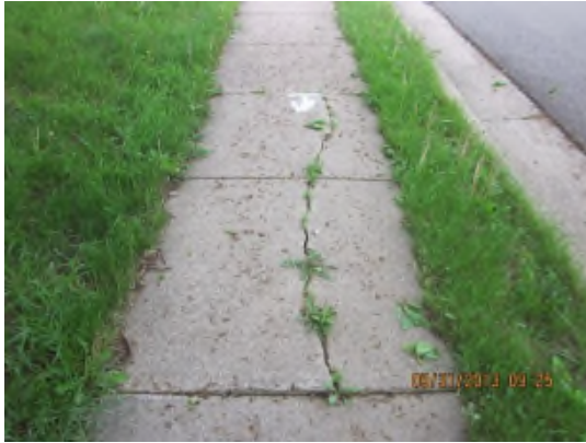
Cracked and heaving sidewalk – Trip Hazard
